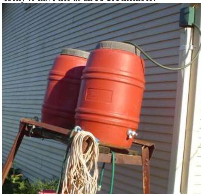
Two Rain Barrels Attached to the Gutter
